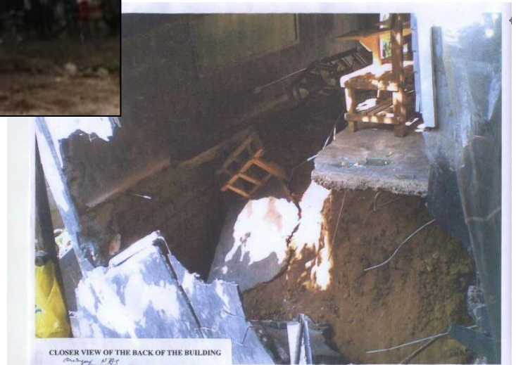
School Building at Aringay National High School in Aringay, La Union that collapsed due to Rainfall-Induced Landslide caused by Typhoon Pepeng.
