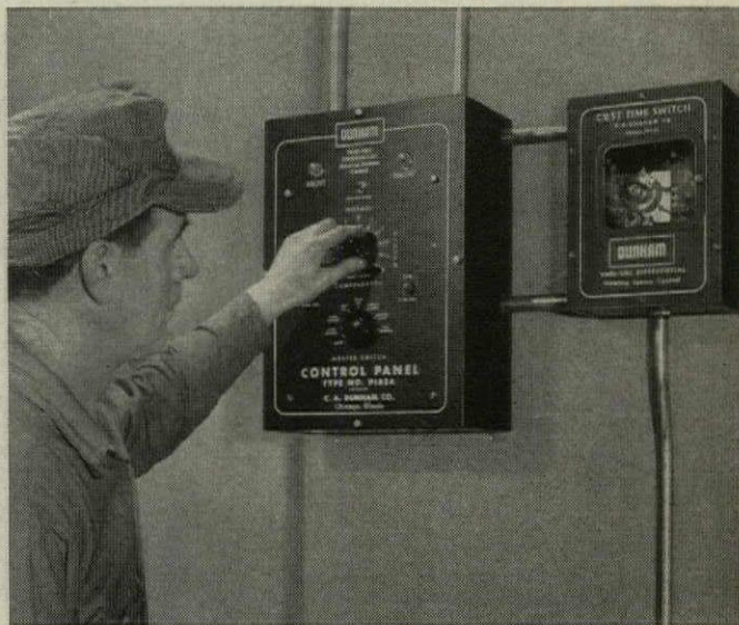
Dunham VARI-VAC Control Panel in Assumption Hall. Provides centralized, one-man operating station for all system settings and remote control readings. The electronic "brain" of this system saves up to 40% on fuel.
