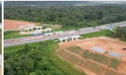
Pembinaan jambatan merentasi Lebuhraya PLUS di Changkat Jering, Perak (Seksyen 11) Construction of bridge across the PLUS Highway in Changkat Jering, Perak (Section 11)
