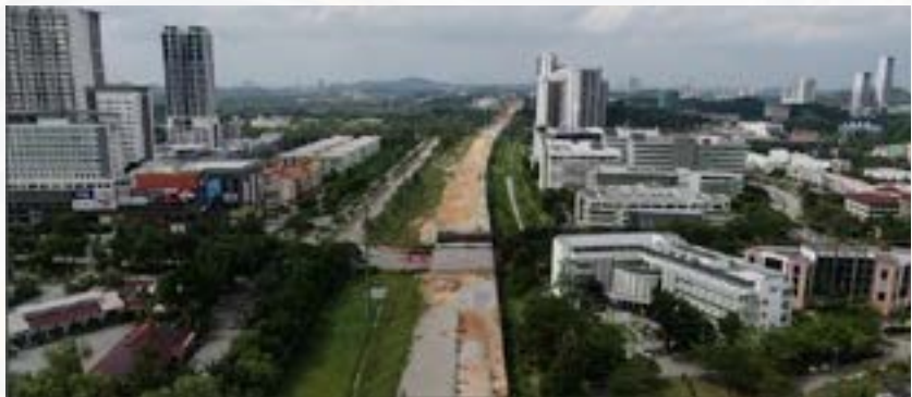
Jajaran Lebuhraya MEX II di kawasan Cyberjaya MEX II Highway alignment in Cyberjaya area
