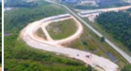
Kerja Pembinaan di Persimpangan Bertingkat Banting (Seksyen 1) Construction Work at the Banting Elevated Intersection (Section 1)
