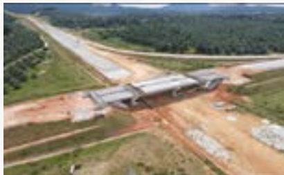
Pembinaan jambatan bagi Persimpangan Bertingkat Trong, Perak (Seksyen 11) Bridge construction for Trong Elevated Intersection, Perak (Section 11)
