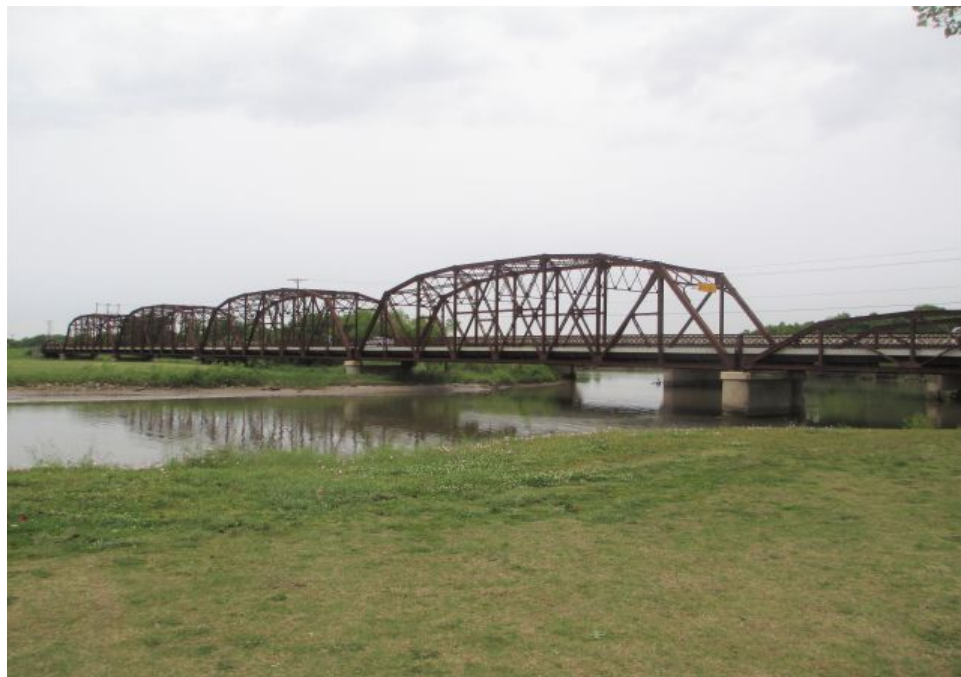
Photo C27. Overview of the original Route 66 alignment over the North Canadian River (see also Resource No. 1 in Appendix A ). View facing northwest.
