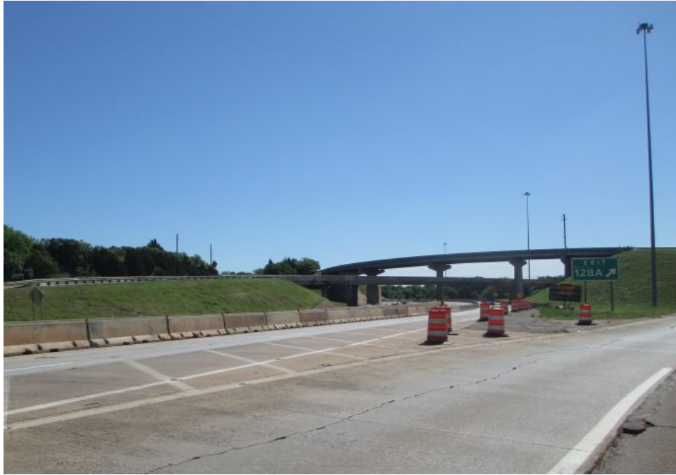
Photo C35. Overview of Lincoln Boulevard and I-44 interchange, which was constructed in 1959. View facing east/northeast.
